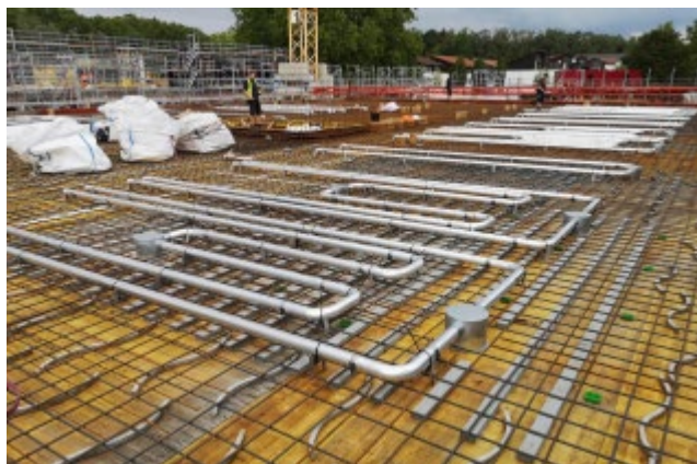
Image 3: Raw ceiling with cooling and heating pipes in combination with Sorp 10® © KaTplan, Münster
